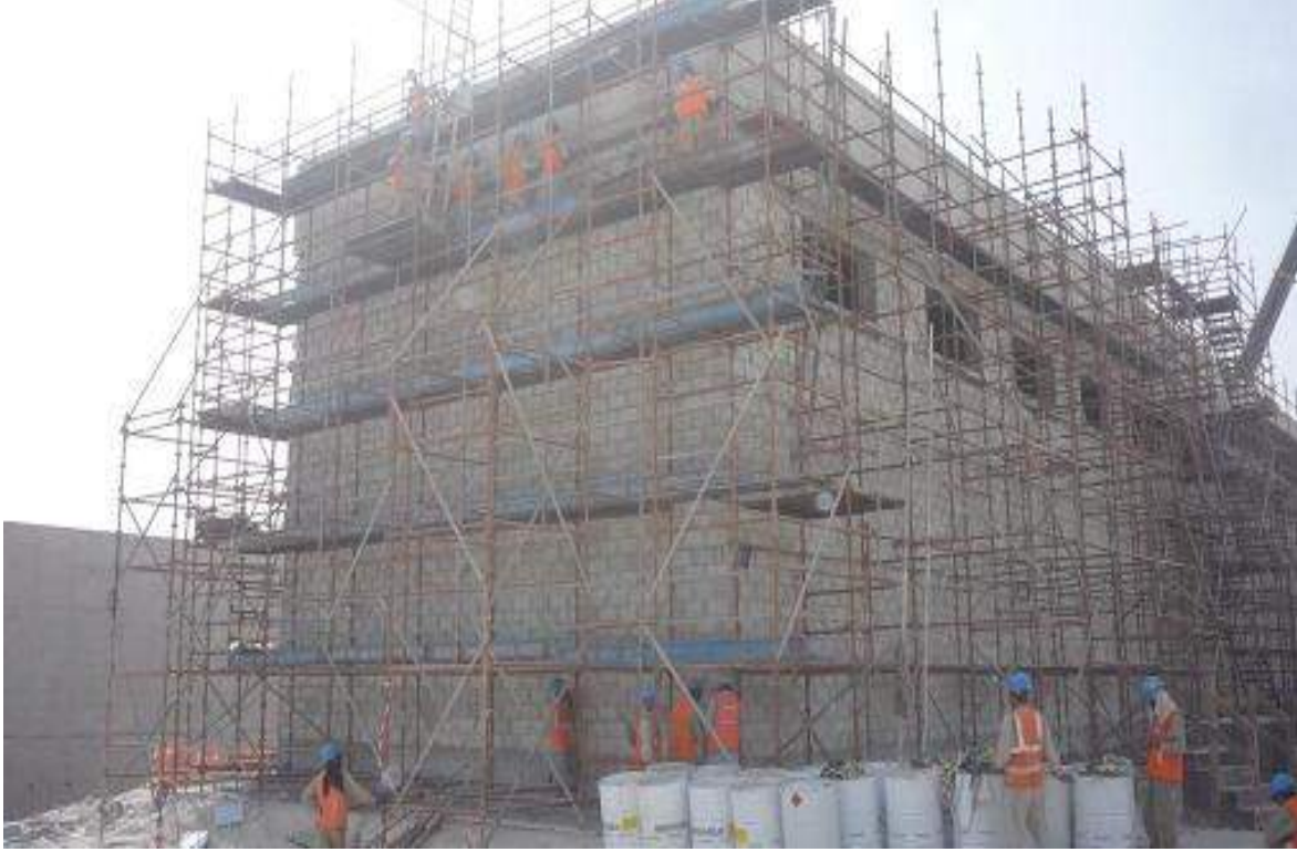
Aeration and MBR Blower Building
