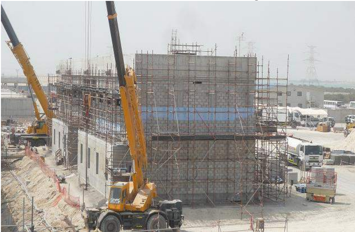
Aeration and MBR Blower Building
